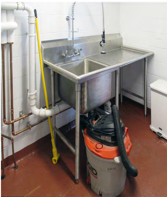
Failure to plan plumbing and bury it in the wall leaves a room impossible to keep clean.
