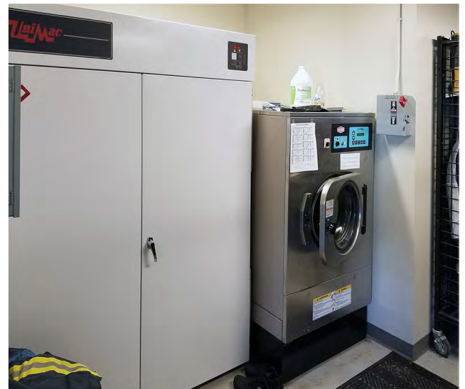
Failure to plan proper spaces in a firehouse's decon laundry area can lead to equipment being installed in a way so that it can't be repaired without the removal of both the disconnect and the machine.
